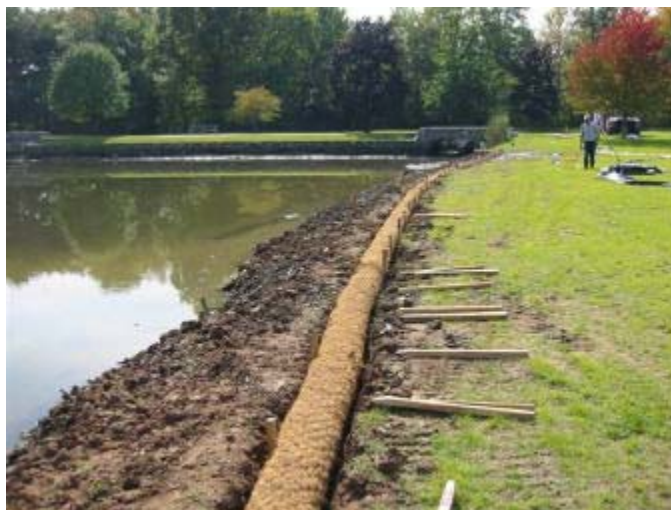
Bioengineering project using fiber roll revetment at Verona Lake, NJ Source: F. X. Browne, Inc.
