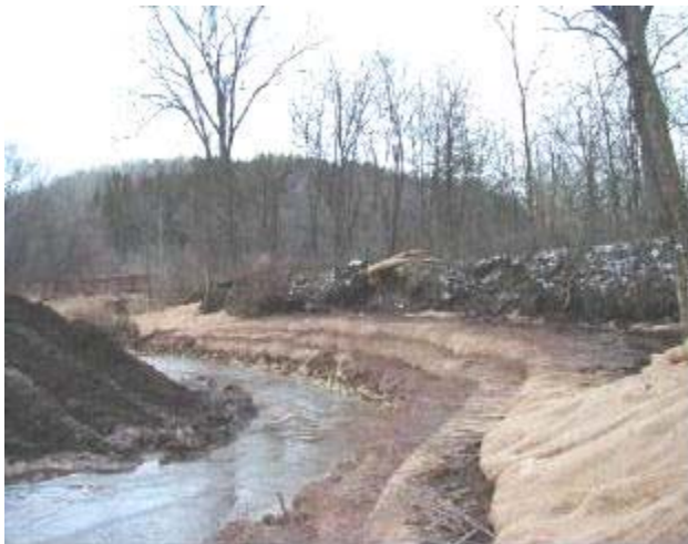
A newly completed vegetated geogrid installation on the Vermillion River, Dakota County, Minnesota Source: Dakota County Soil and Water Conservation District
