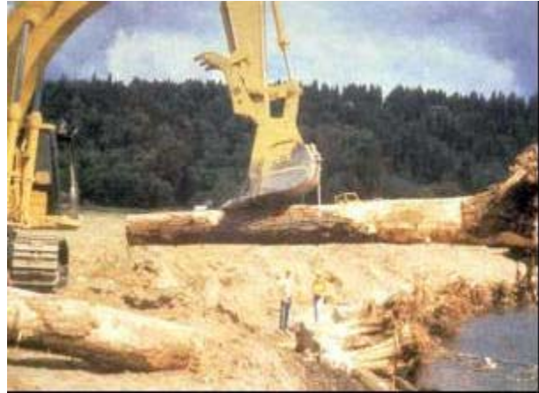
A track hoe is used to lower a large rootwad into place
