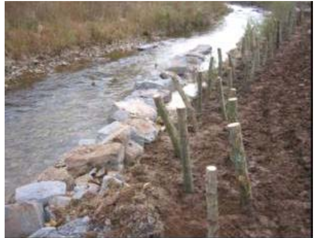
J-hook rock vane and dormant post installation in Cooks Creek, Bucks County, PA. Source: F. X. Browne, Inc.
