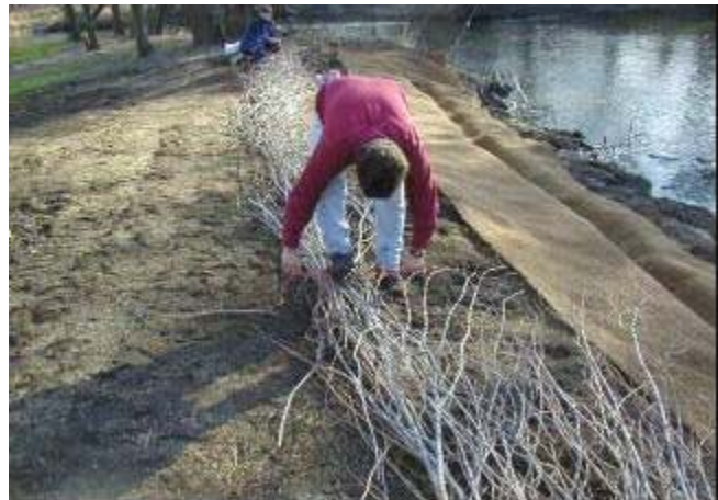
Preparing live material bundles for a live fascine installation. Note the erosion blanket-lined trench awaiting bundle placement. Source: Dakota County Soil and Water Conservation District
