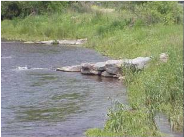
Rock vane installation along Martin's Creek, Northampton County, PA. Source: F. X. Browne, Inc.
