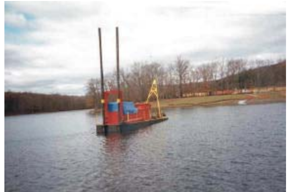
Hydraulic dredging: A typical dredging barge equipped with a cutterhead dredge. Source: F. X. Browne, Inc.
