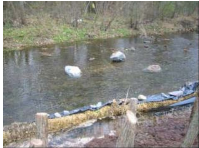
Boulder placement for habitat enhancement along a stretch of Cooks Creek, Bucks County, PA
