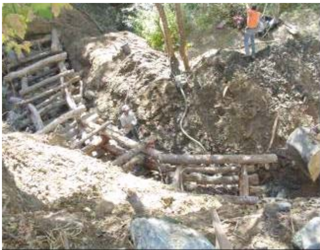
Installation of a cribwall structure during the Palomares Creek Streambank Restoration Project Source: Alameda County Resource Conservation District
