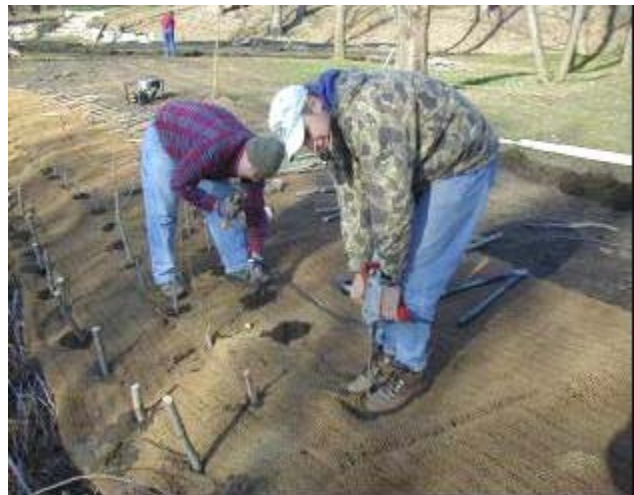
A two-man crew installs live stakes along the Vermillion River, Dakota County, Minnesota
