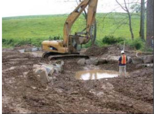
Construction of a cross-vane structure and downstream scour pool for a natural channel design project
