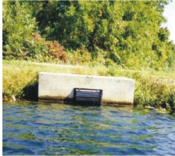
Fish escapement device installed on outlet structure of a pond in Snyder County. Source: Edward Molesky of Aqua-Link, Inc.
