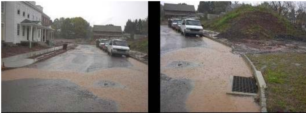
Sediment-laden surface runoff generated at an active construction site (left). Surface runoff flowing into storm drain, which discharges directly into nearby stream (right). Source: Edward Molesky of Aqua-Link, Inc.
