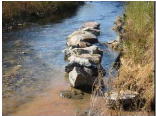
Vane rocks are placed starting from the vane tip back towards the streambank. Source: F. X. Browne, Inc.
