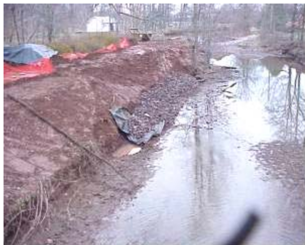
Boulder toe installation along a streambank stabilization project in Perkasio Borough, Bucks County, PA Source: F. X. Browne, Inc.
