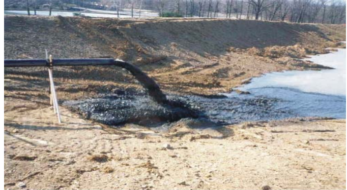
Sediment slurry inflow into a sediment disposal basin for a hydraulic dredging project.
