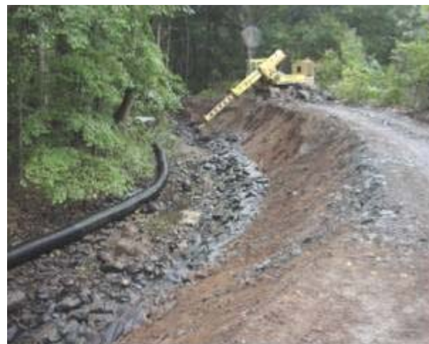
Installation of a Boulder toe along Sambo Creek, Monroe County, PA Source: F. X. Browne, Inc.
