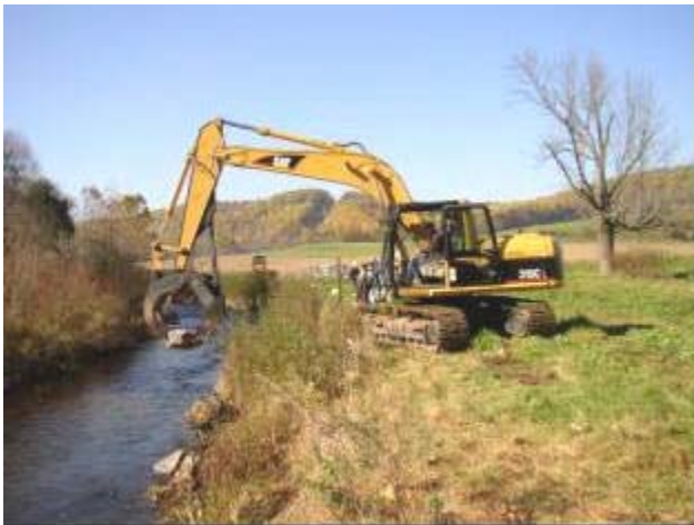
A track hoe with a grapple attachment is used to place vane rocks for a J-hook rock vane installation on Cooks Creek, Bucks County, PA. Source: F. X. Browne, Inc.
