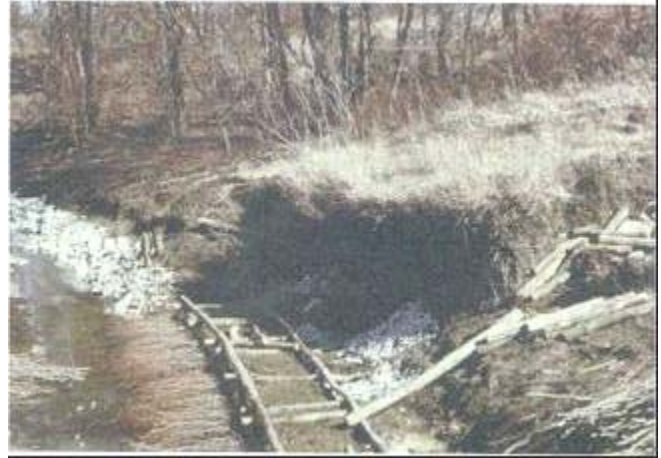
Installation of the first course of timbers and live material in a live crib wall
