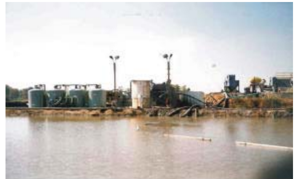
Hydraulic dredging: mechanical dewatering equipment used to dewater sediment slurry in place of a sediment disposal basin
