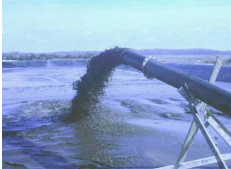
Inflow pipeline from a hydraulic dredging operation discharging dredged material into the disposal basin. Lake Lily, NJ. Source: F. X. Browne, Inc.
